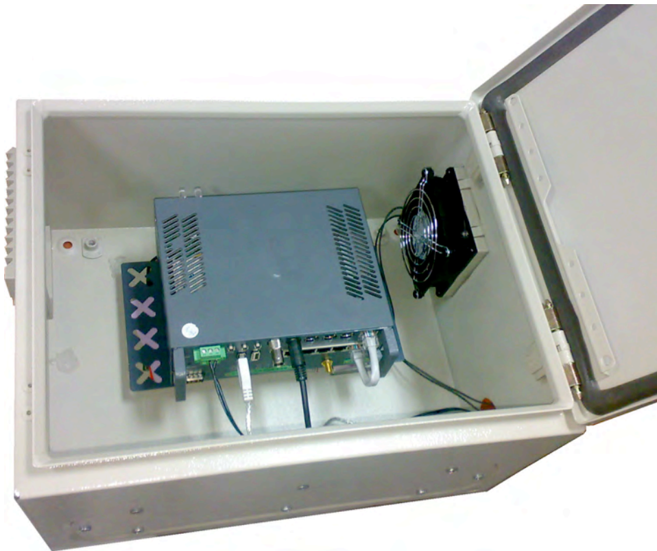
Figure 1: TVG unit installed in an insulated container
